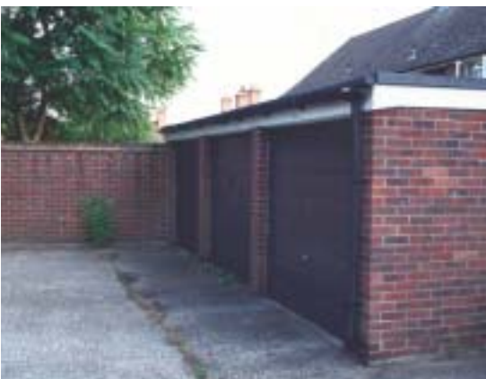
Rear parking – Poor surveillance, poor quality
